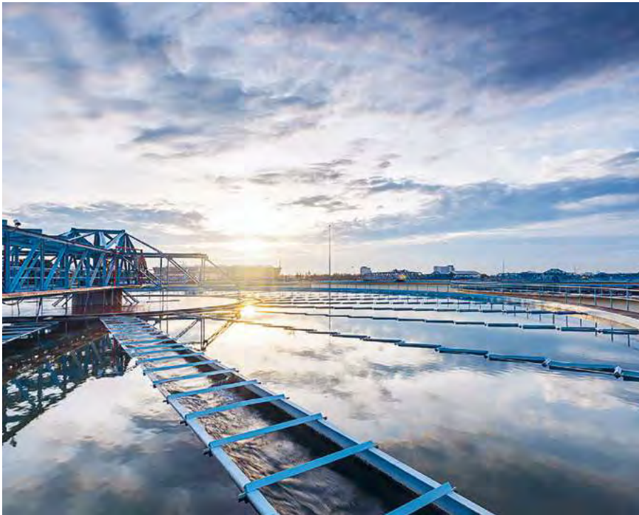
Water treatment is an essential element of every metallurgical plant.
